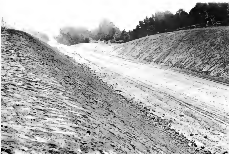
Cut slopes, 1\frac{1}{2} :1 that were blanketed with 6 inches of top soil as part of contract
